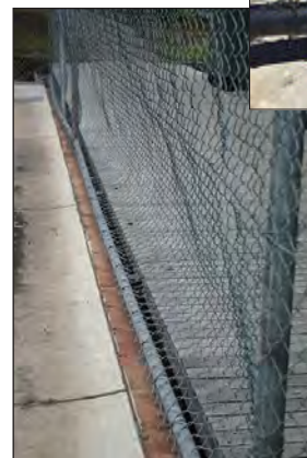
Sagged chain-link on Club court accentuated by support rails too close.
